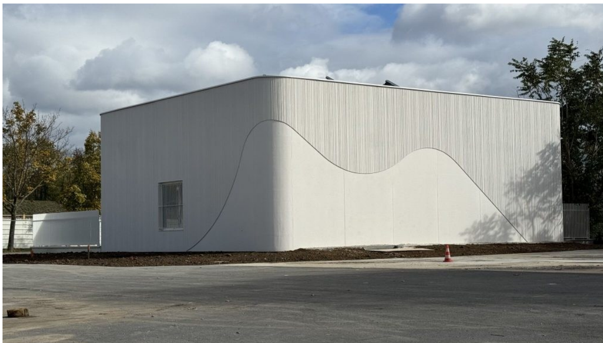
Figure 5 The exterior of the geothermal heating plant at Fort de L'est in Saint-Denis, France
